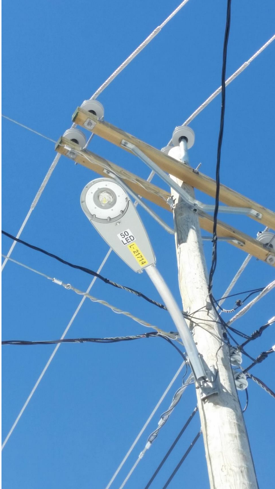
Photo above: New LED Streetlight
